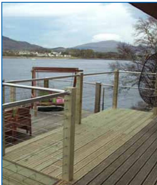
Wire Rope System
